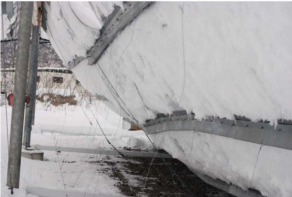
Figure 4.1: The snow collected and created square icicles which hung below the mesh adding weight to what was already collecting above.
