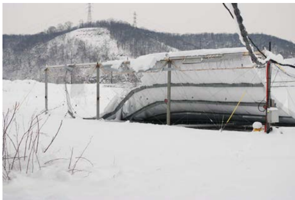
(a) Partial collapse of the east cylinder.
