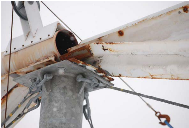
Figure 4.9: The truss twisted and was torqued when the mesh fell instead of being under pure compression.
