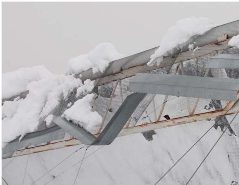
Figure 4.7: The finger plates also ended up being a point of failure. They bent and tore through the mesh.
