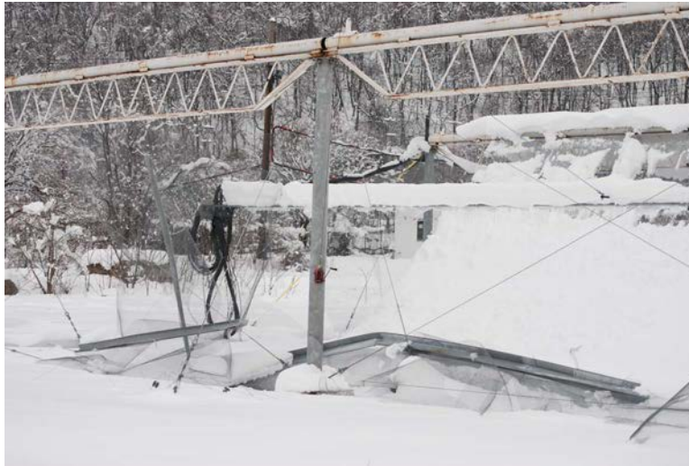
Figure 4.8: The West cylinder seemed to fail differently. The northwest end had fence wire failures. The rest of the cylinder failed at the mesh right above the top batten.
