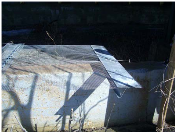
(b) mesh beginning to tear
